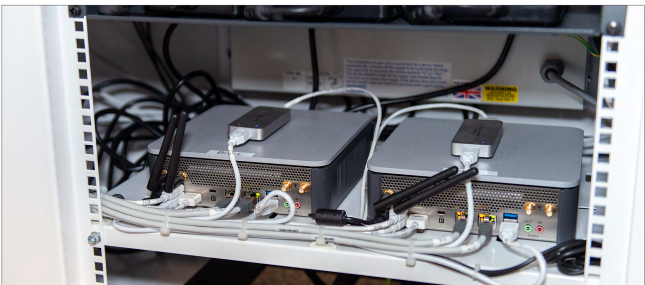
Two Cynap Cores are installed at each workstation. Magewell USB Capture HDMI frame grabbers are used to provide the additional option of wired HDMI input connectivity at each workstation.
