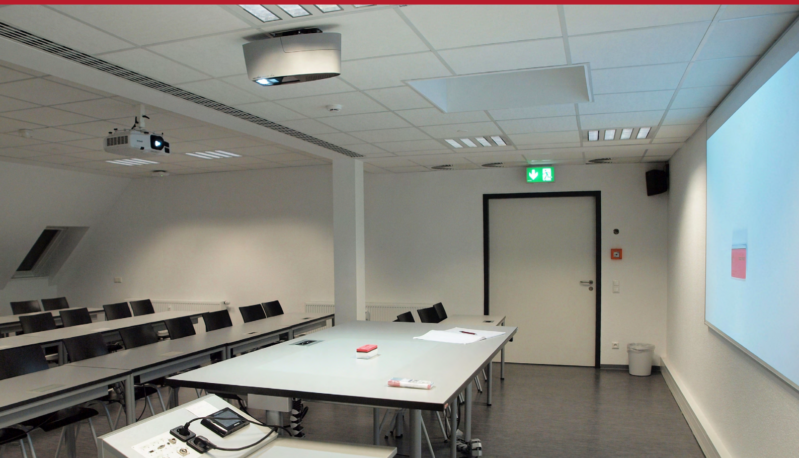
At the University of Siegen, Faculty III, two rooms were equipped with WolfVision VZ-C6 Ceiling Visualizer systems.
