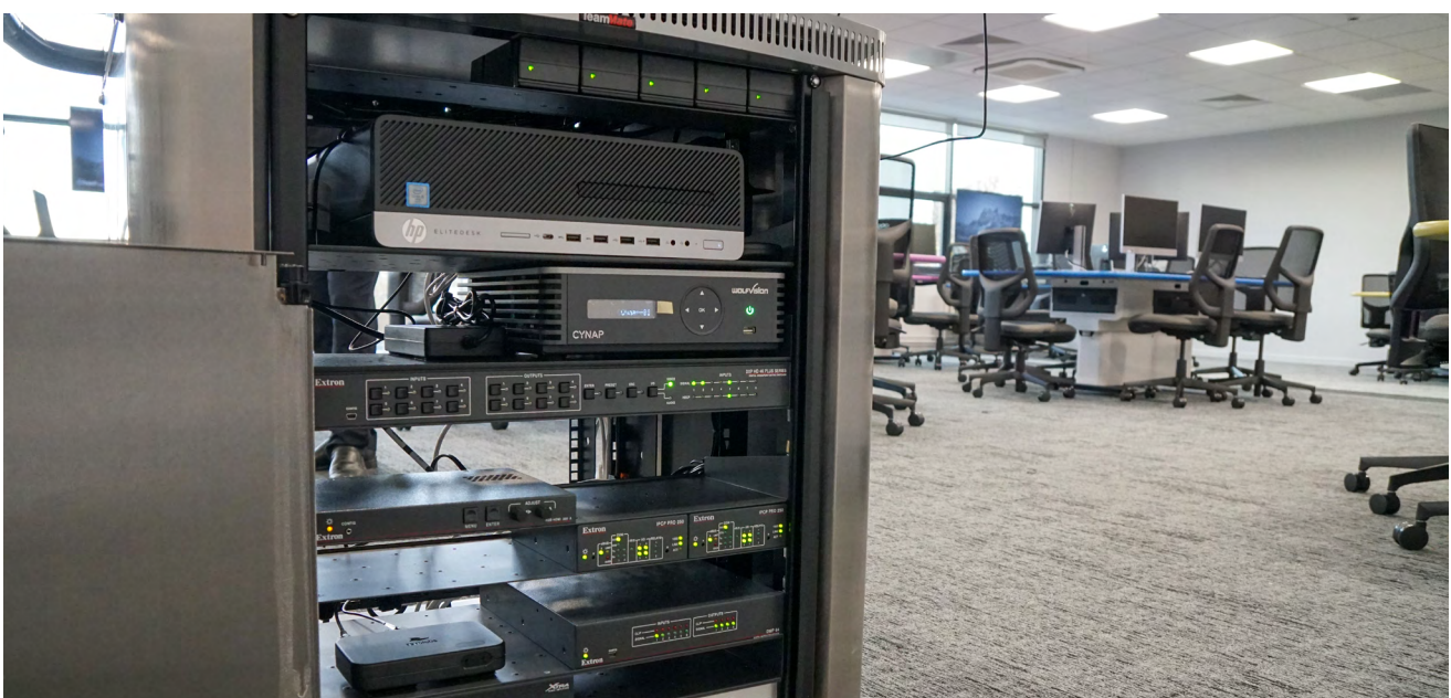
Main Cynap unit with vSolution MATRIX-enabled feature pack, installed in the 19”rack of a TeamMate Educator lectern.
