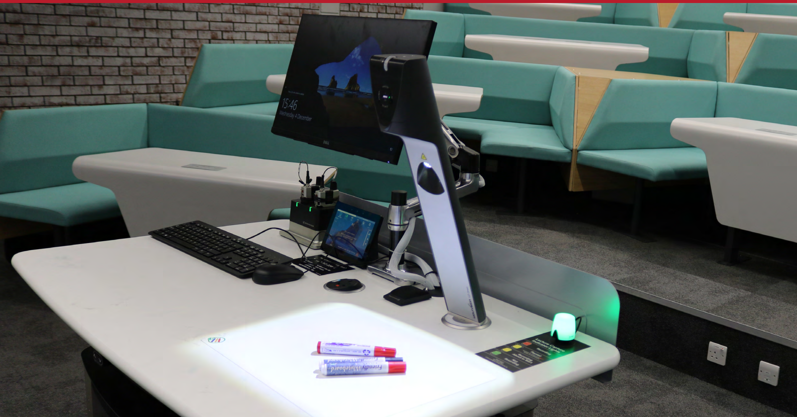
WolfVision Visualizer installed on the lectern, enabling high quality on-screen display of handwriting and objects of all kinds at The University of Warwick.
